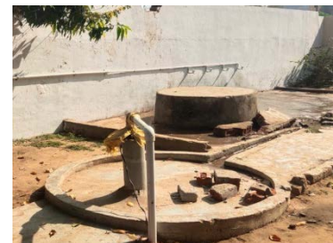
Constructed a tank to facilitate drinking water facility at Primary School, Ravipura; aided by Sardar Patel University
